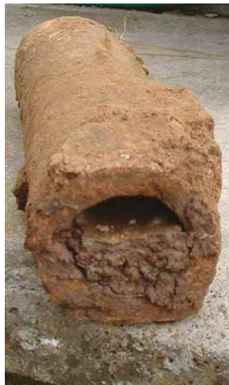
Figure 22. Silted clay drain
