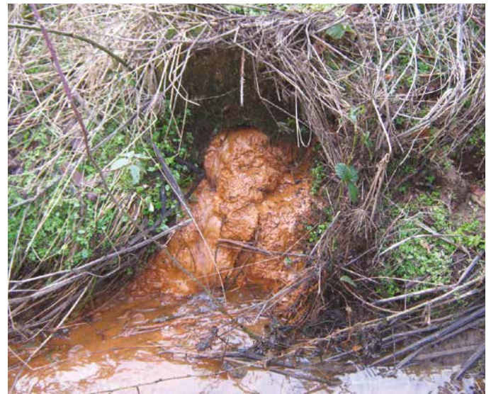
Figure 24. Drainage outfall blocked by ochre
