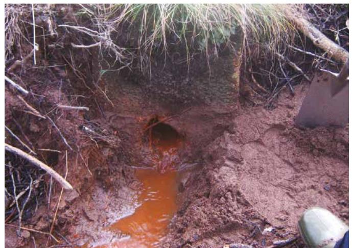
Figure 21. A blocked outfall can often be cleared in a matter of minutes with a spade
